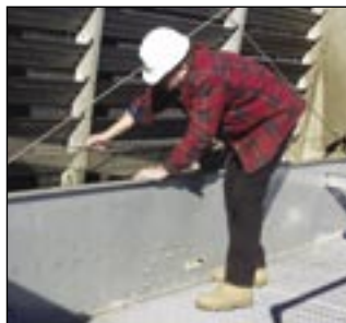
Cold water basin strainer.
