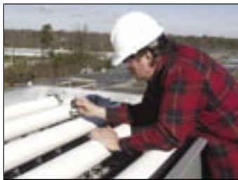
Spray distribution nozzles.
