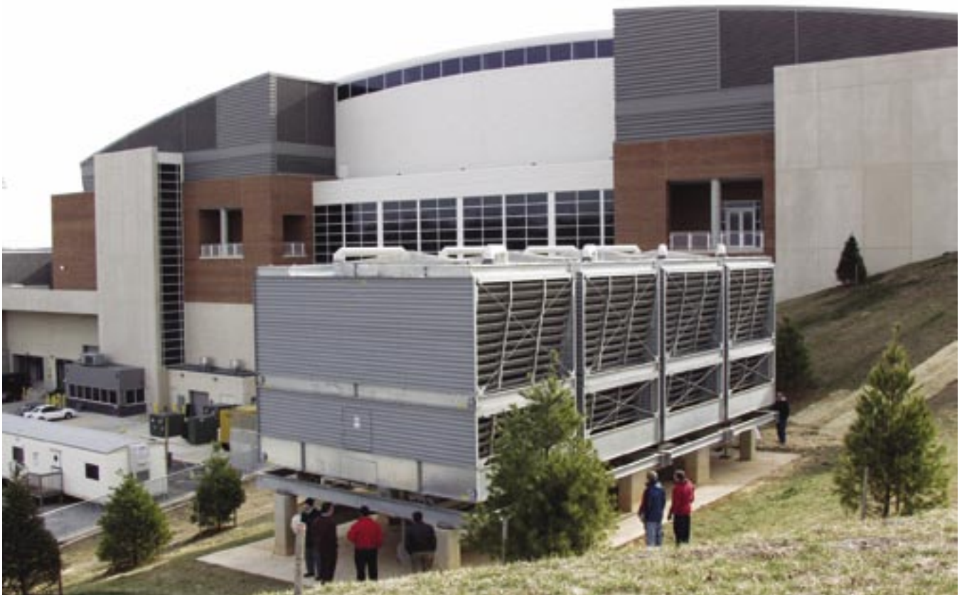
Cooling towers away from the building can be subjected to the “out of sight, out of mind” principle.
